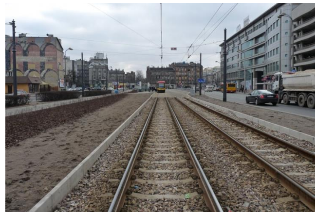
Fig. 1 One of the modifications of the rail fastening of SB-3 type used for tram tracks in Warsaw
