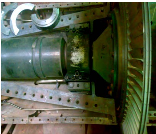
Fig. 2 Rotor failure in examined gas turbine
