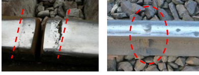
Fig. 1 Rail defects: Insulated rail joint with wide gap (left) and rail weld (right)
