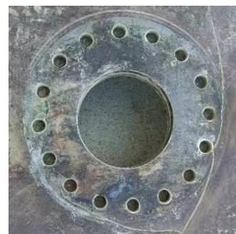
Fig. 13 Ductile cracks of side plan
