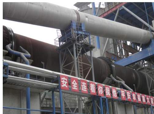
Fig. 1 Rotary kiln in a cement plant of China
