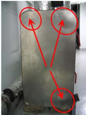
Fig. 3 Defects on brazed plate type HE due to pressure influence of heat transfer media after two years of exploitation
