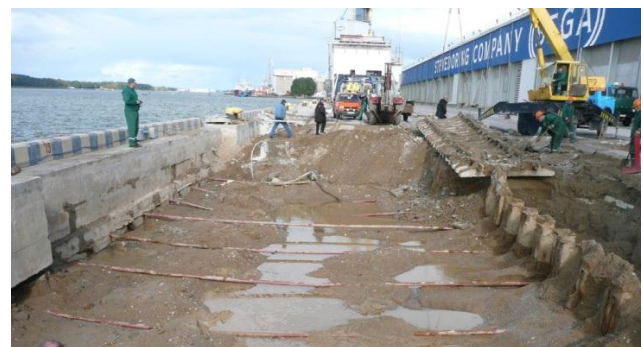
Fig. 9 Real situation of quay wall with anchors and VHP columns (after excavation)
