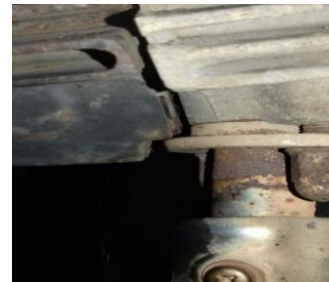
Fig. 1 Crack due to lack of fusion and visible result of corrosion
