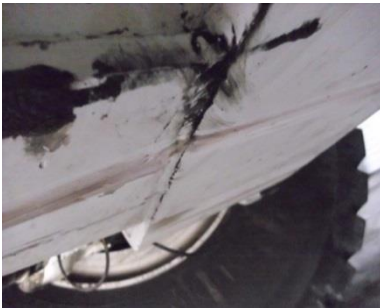
Fig. 1 Visible Welding seam cracks of A-type frame
