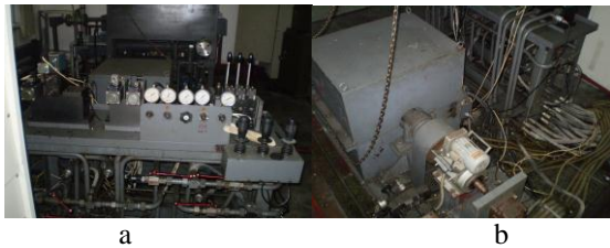
Fig. 20 Valve group of the system (a) and simulation load equipment (b)
