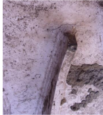
Fig. 10 Cracks at root of the ear plate in right rear suspension support
