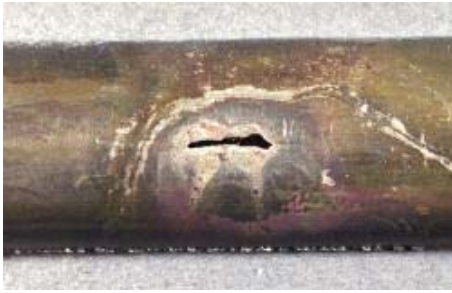
Fig. 2 Outside surface of the damaged connecting tube due to corrosion influence
