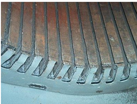
Fig. 1 A loose stator stack [3]
